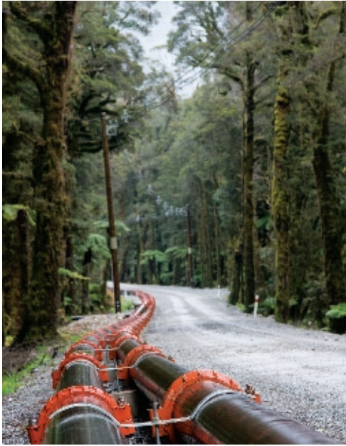
Coal slurry pipeline winding through trees
